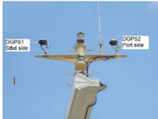
Good Installation – Antenna at Top of Mast with Good Spacing
