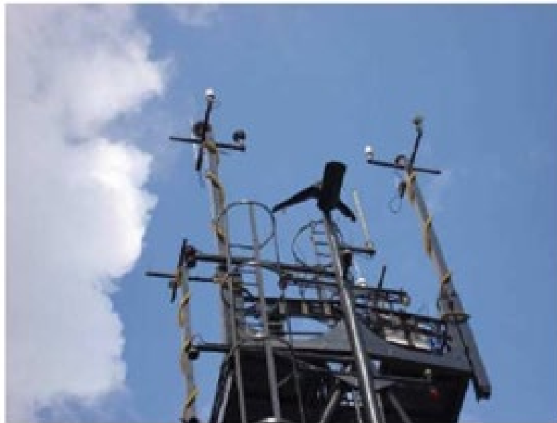
Good Installation – Antenna at Top of Mast with Good Spacing
