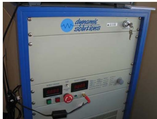
Figure 2 DS2200 Control Panel
